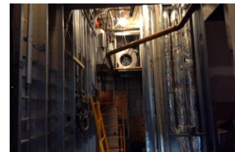
Antenna cables snake through the building ...
